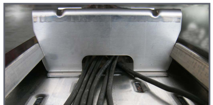
Floor rail used as a cable duct for the string cables
