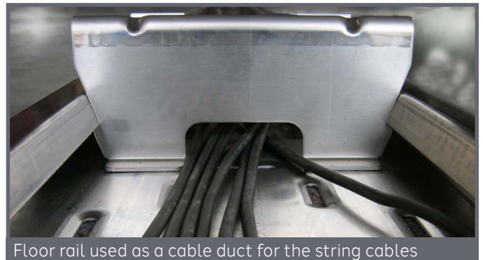
Floor rail used as a cable duct for the string cables
